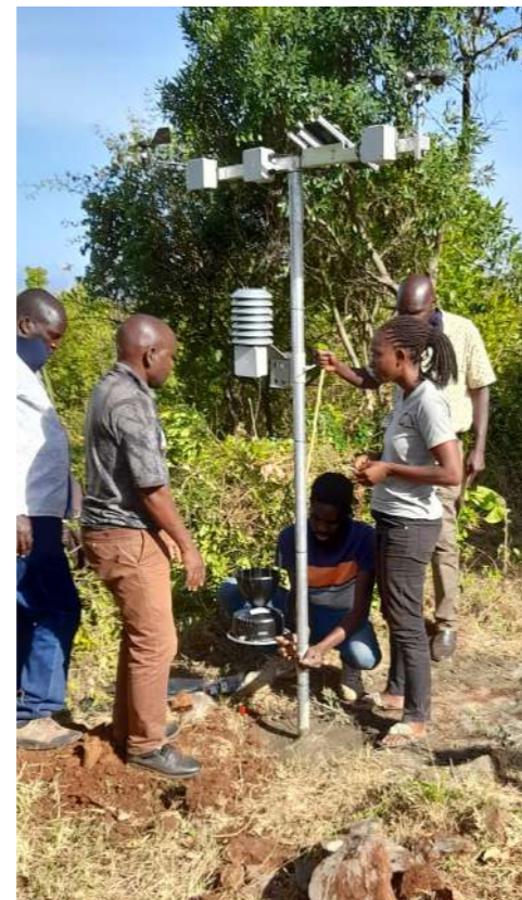
Installation in Bukwo district
